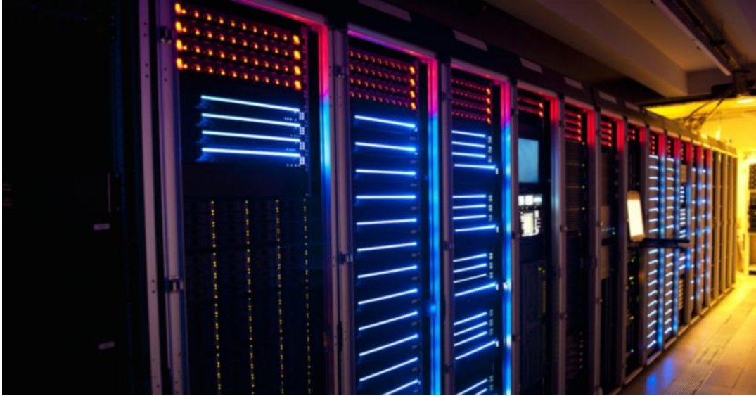
Figure 2: Infrastructure: Data Center
